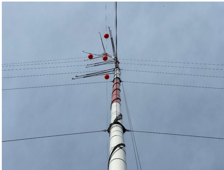
Figure 1: Damage MET Tower
