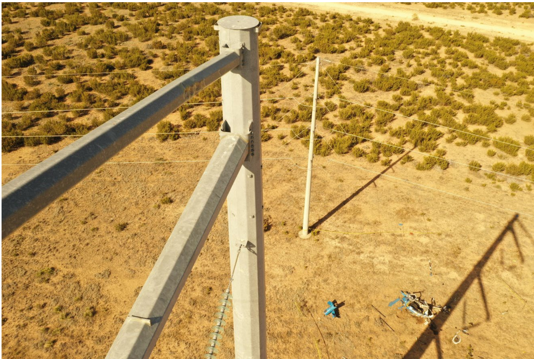
Photograph 1 - Aerial view of the static arm that was impacted by the helicopter (courtesy of Brim Aviation)
