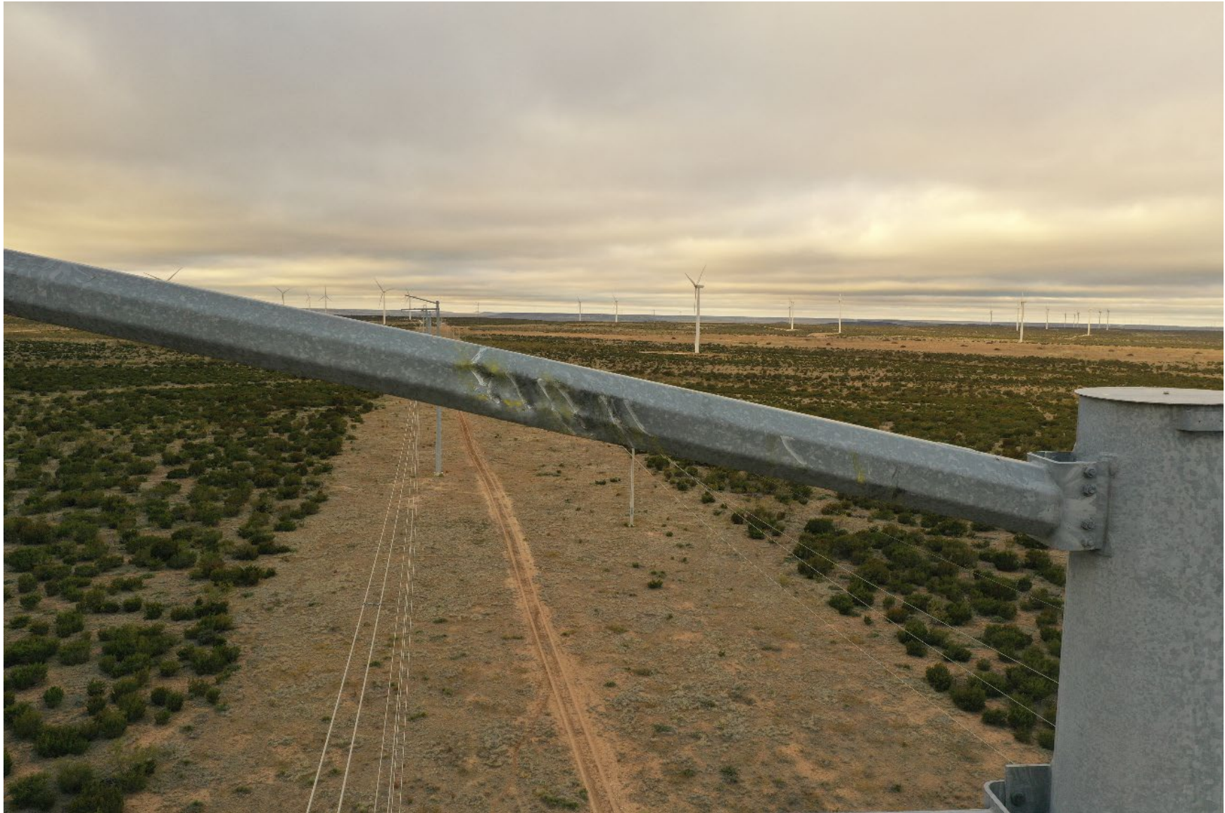
Photograph 2 - Aerial view of the static arm that was impacted by the helicopter (courtesy of Brim Aviation)
