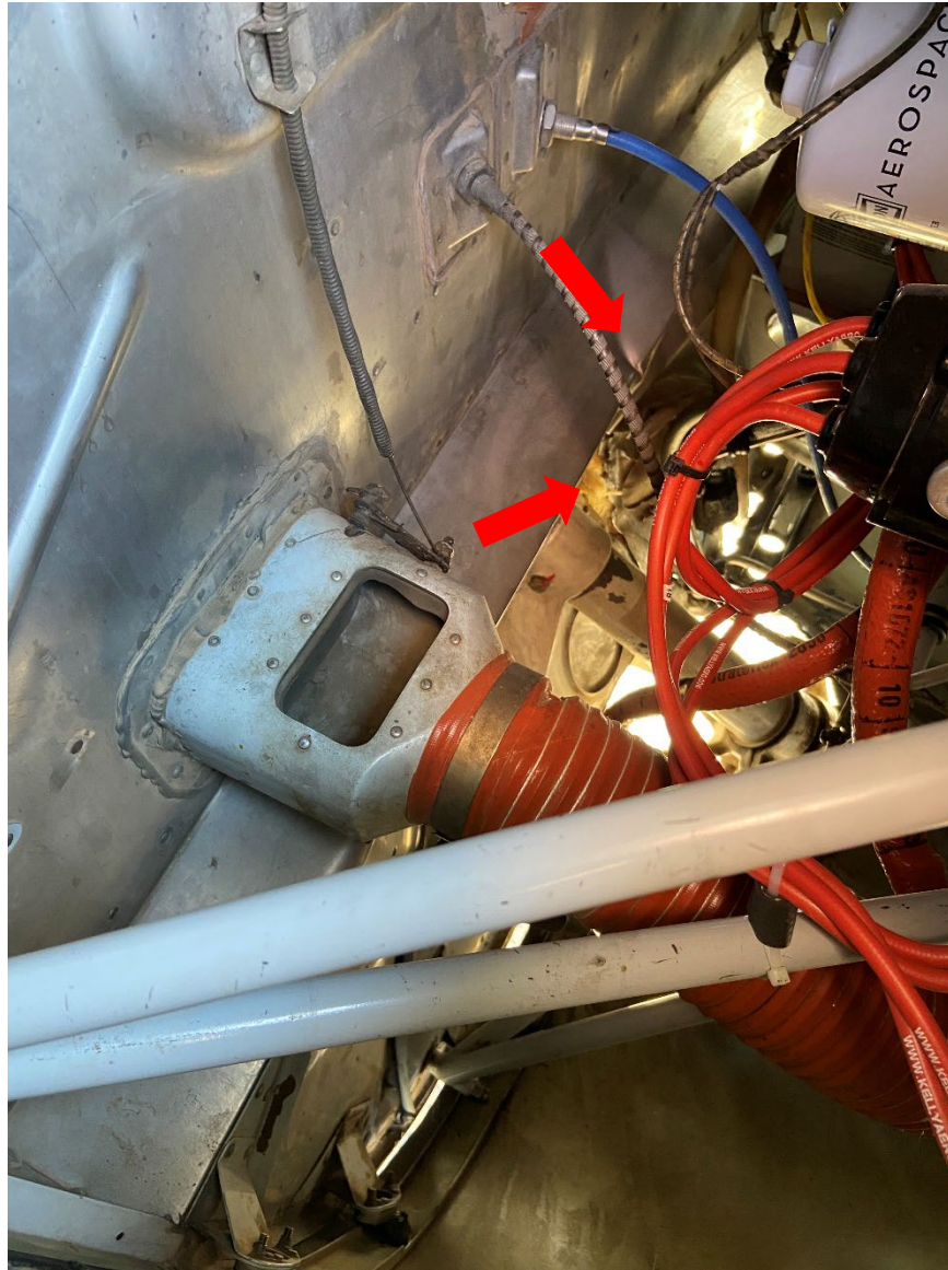
Photograph 2 - Damaged Upper and Lower Firewall (Courtesy of FAA)
