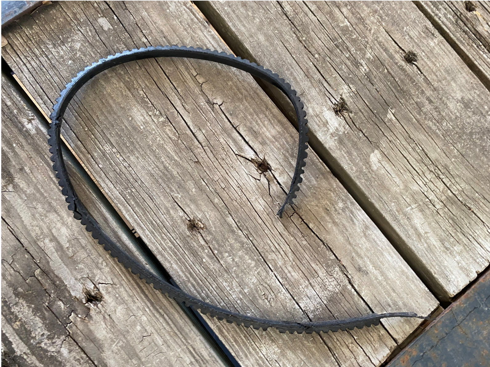
Photograph 5 - Broken belt from alternator No. 2 (Courtesy of FAA)
