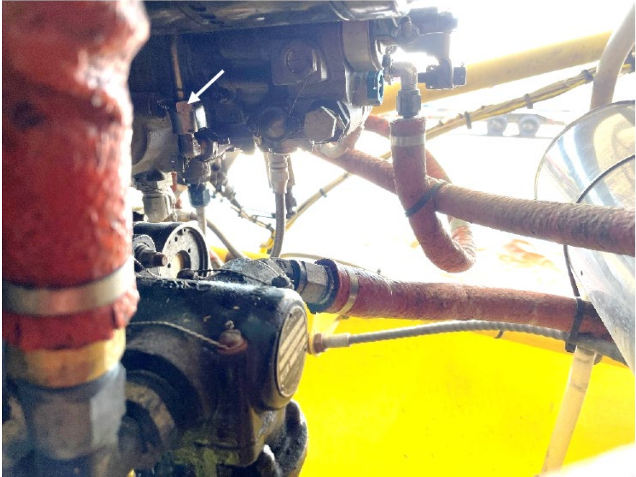
Figure 17 - Py Fitting at FCU
