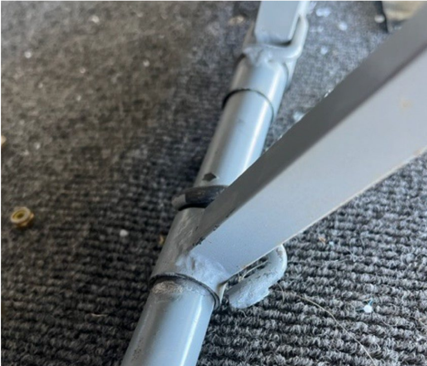
Photograph 9 - Failed weld (Courtesy of FAA)
