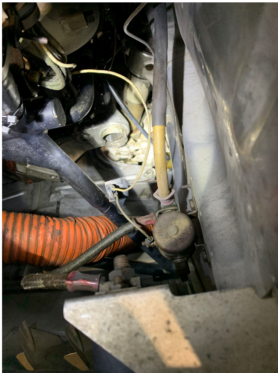
Photo 1 – Firewall damage. (Photo courtesy of FAA)
