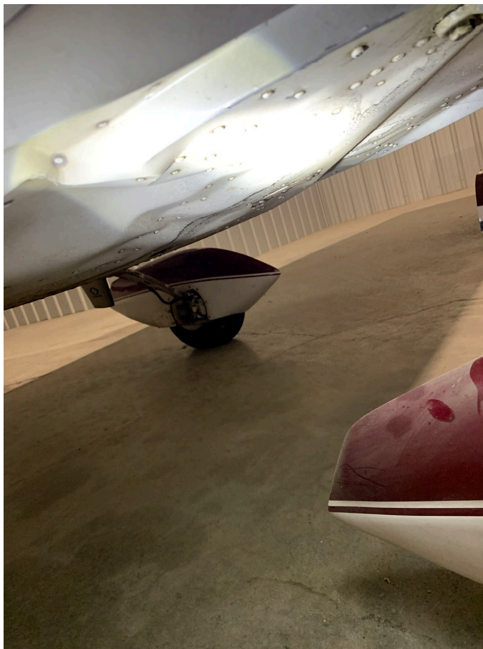
Photo 2 – Bottom of forward fuselage showing skin buckling. (Photo courtesy of FAA)
