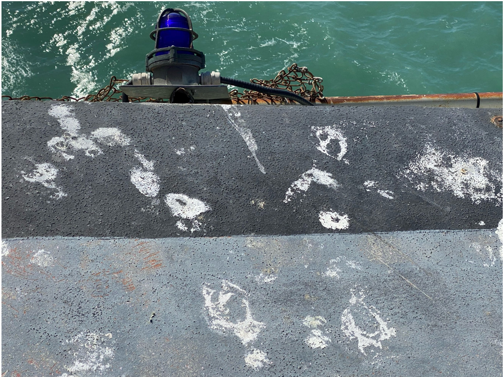
Photo 5 – Platform skirting and light damage (Source: Rotorcraft Leasing Company)
