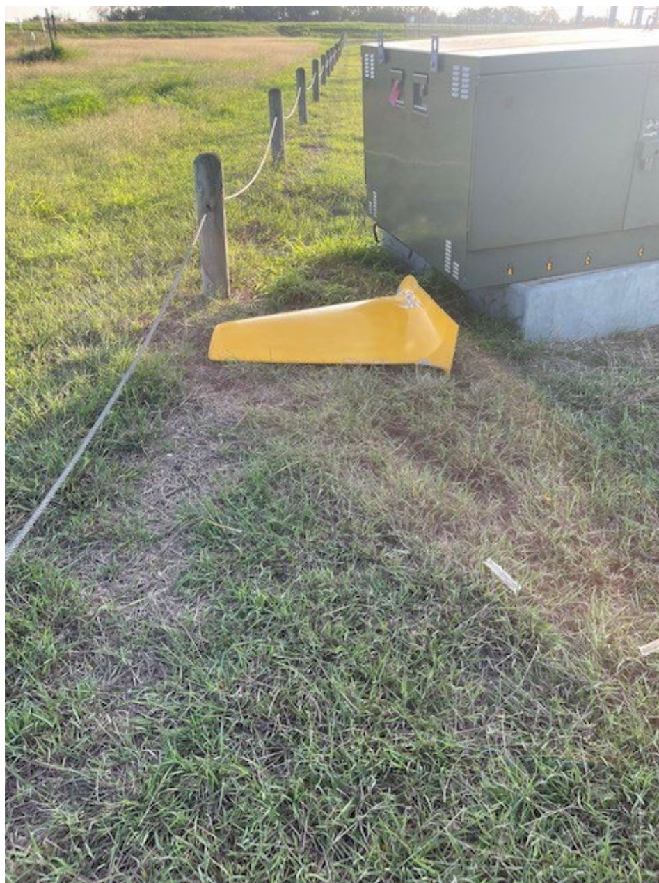
Photo 4: Damaged winglet / electrical box – (Photo provided by FAA)
