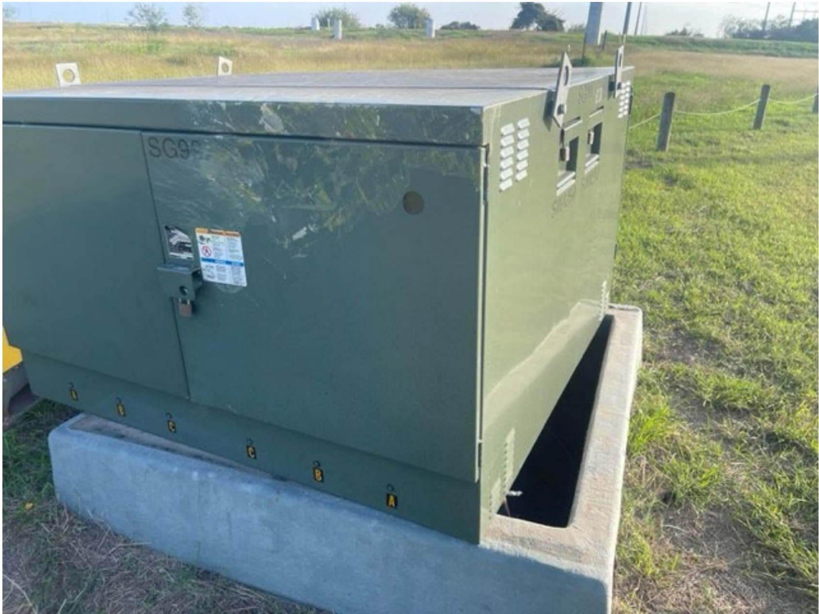
Photo 3: Electrical Box / Moved off the foundation and yellow paint transfer – (Photo provided by FAA)
