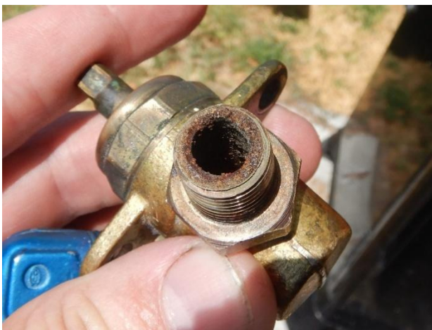
Figure 8. Outlet of fuel shutoff valve
