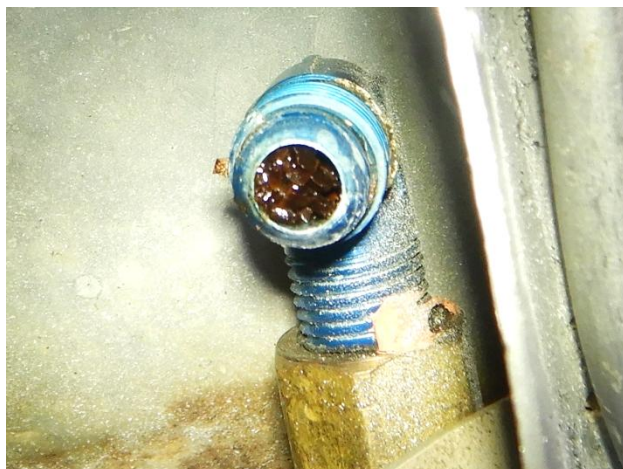
Figure 7. Inlet to fuel shutoff valve
