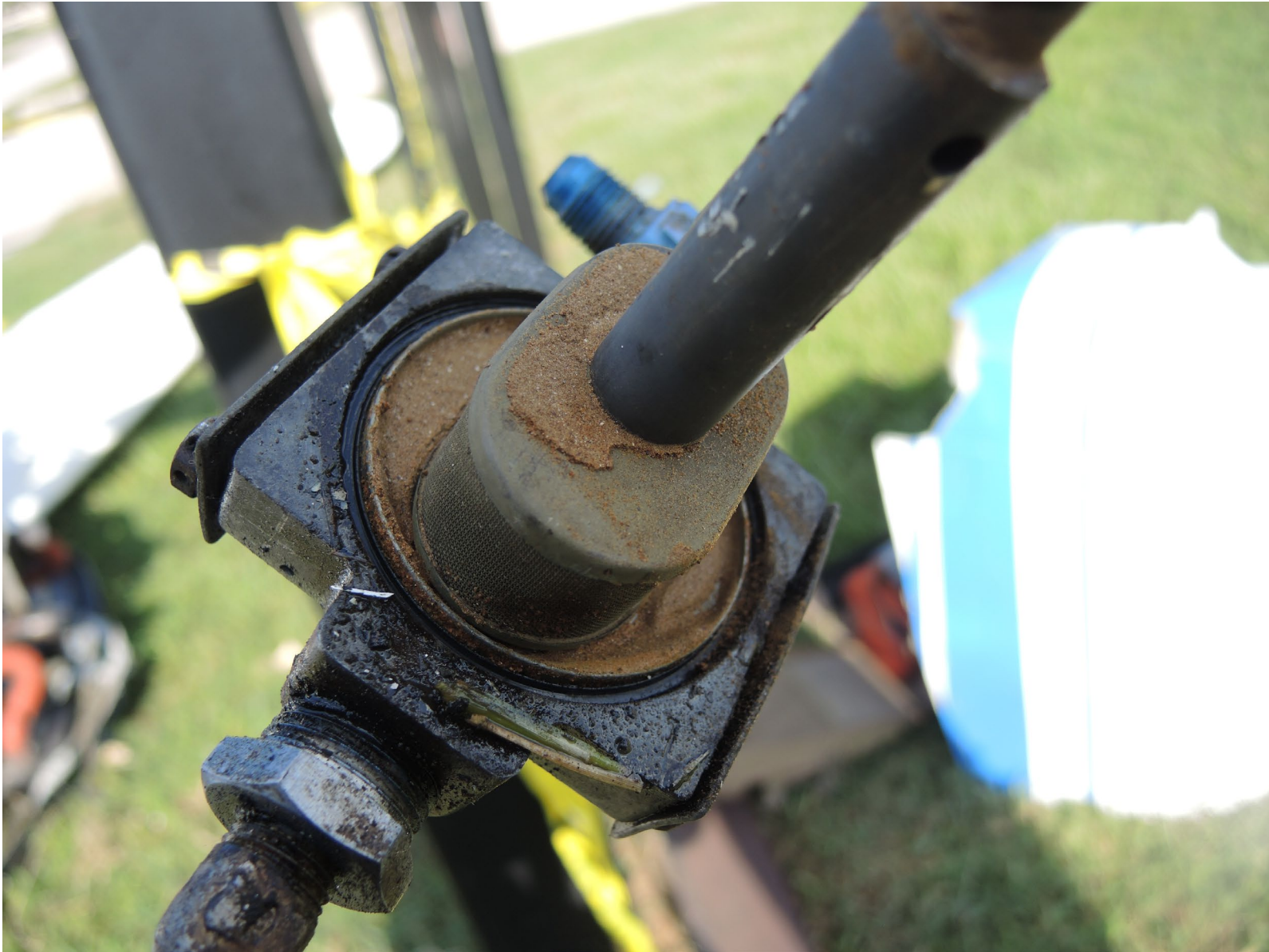
Photograph 10 - Debris in fuel strainer
