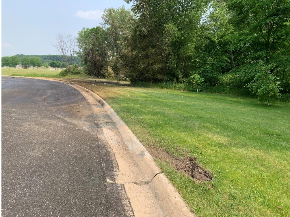
Figure 1. Initial impact location at concrete curb and asphalt road
