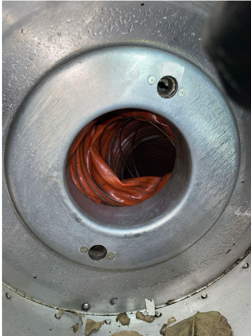
Photograph 3 - Partially collapsed induction hose (NTSB Photo)
