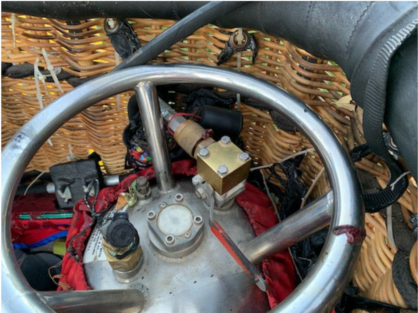
Photo 5 – Top of Propane Tank / Fittings / Burn Indications (Photo Provided by FAA)
