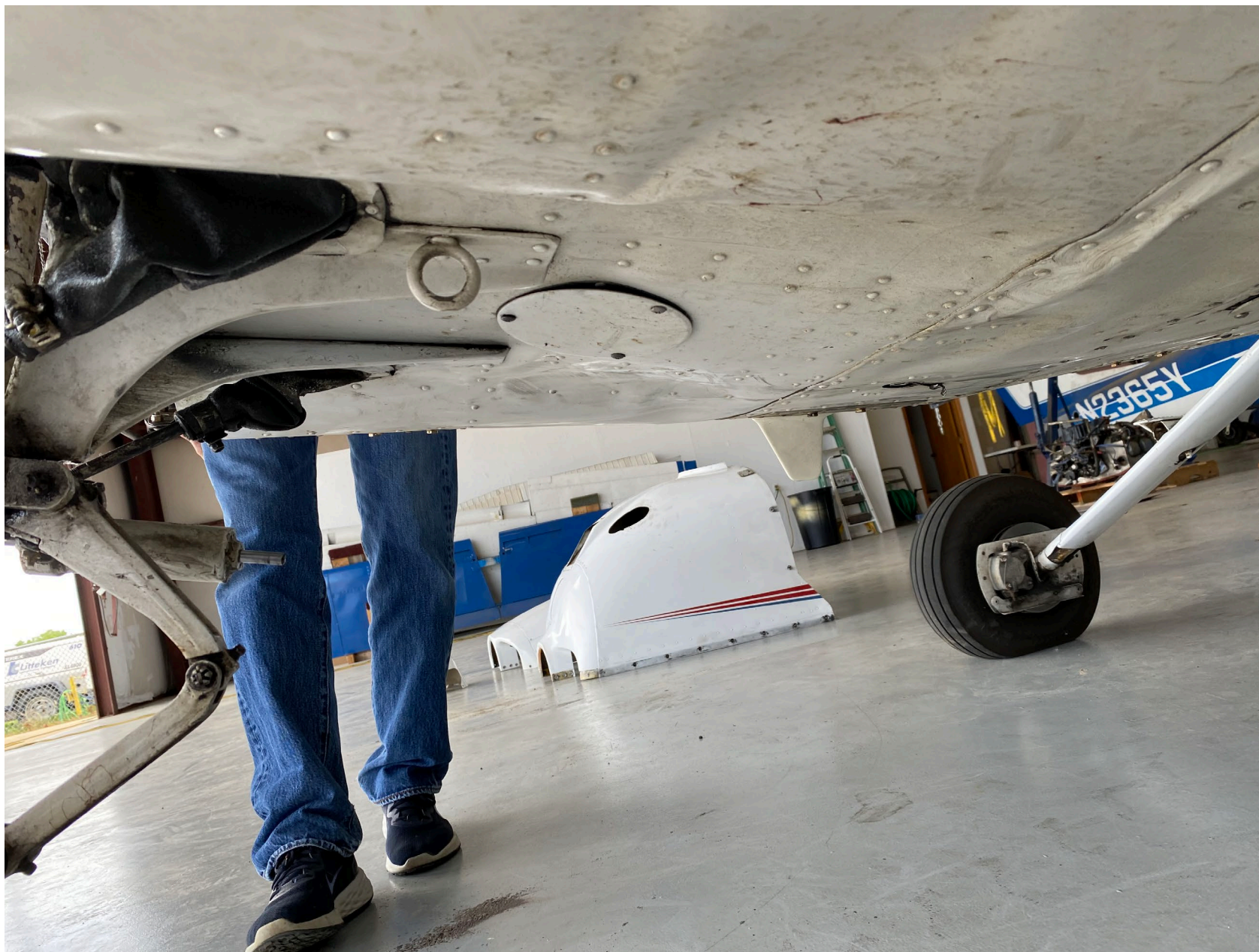
Photo 3 – View of the damage sustained to the underside of the fuselage (courtesy of the Federal Aviation Administration).
