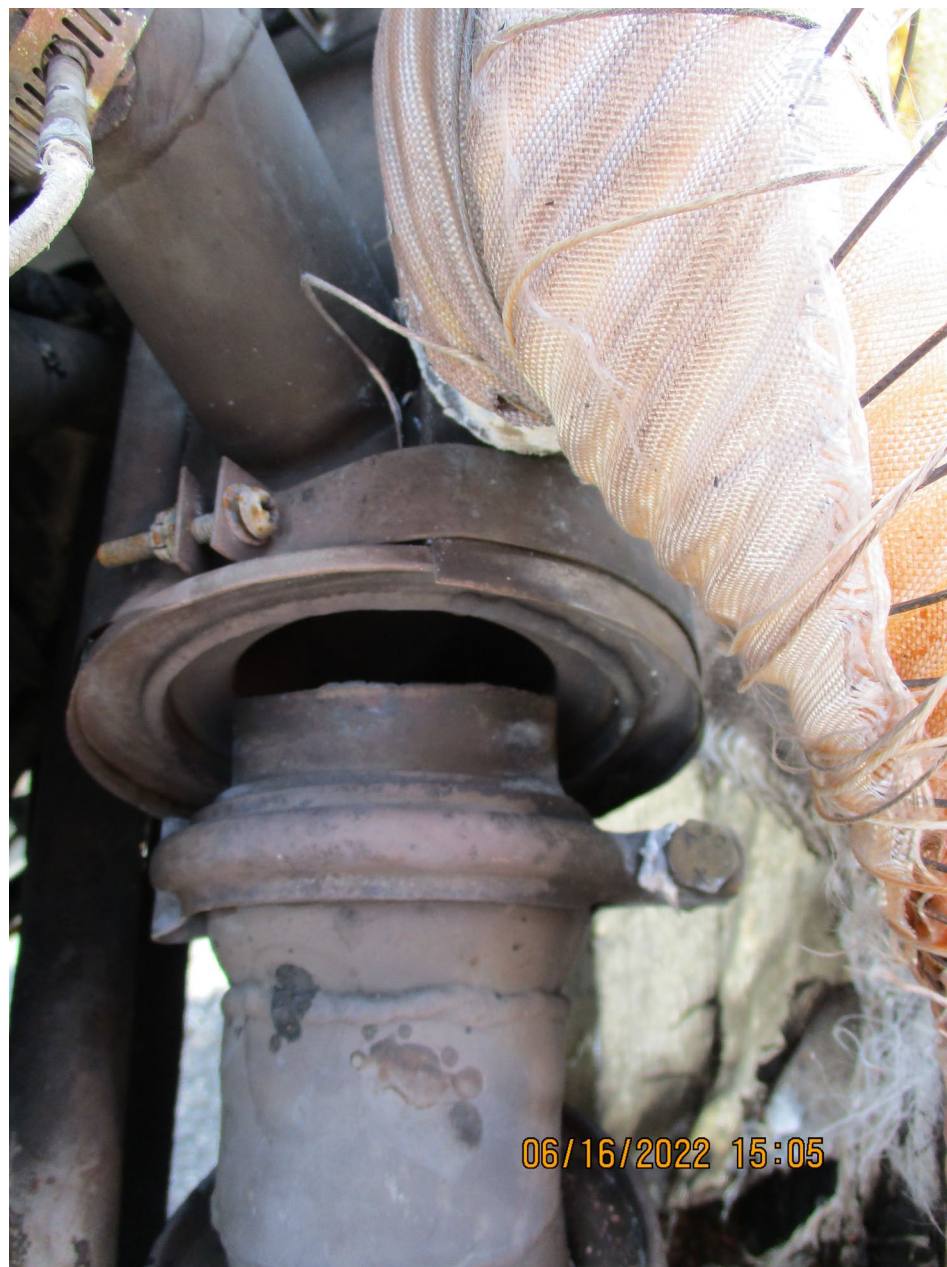
Photo 3 – Exhaust Components at Initial Exam, Courtesy of FAA
