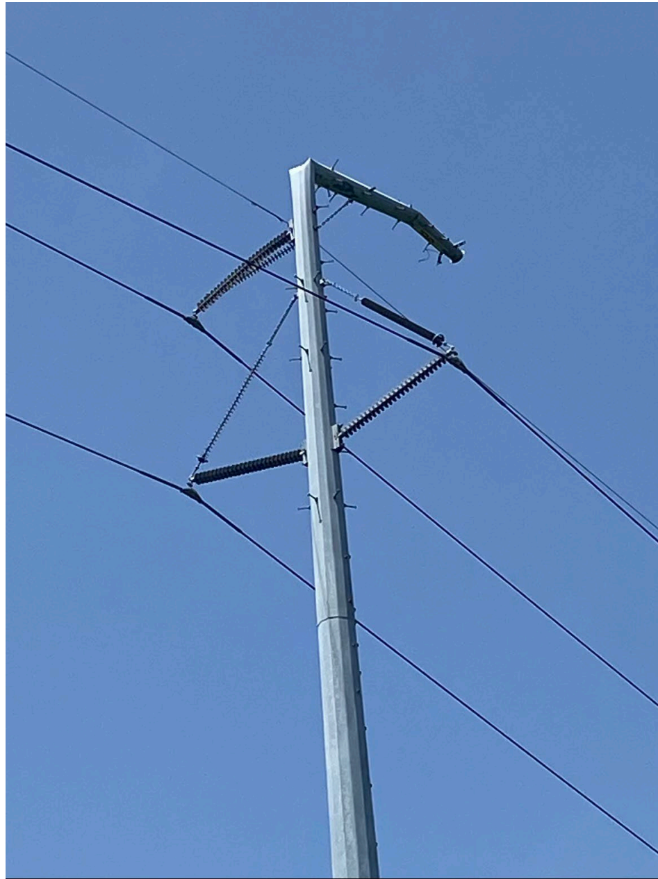
Photo 3 – Power Line Pole – Courtesy of FAA
