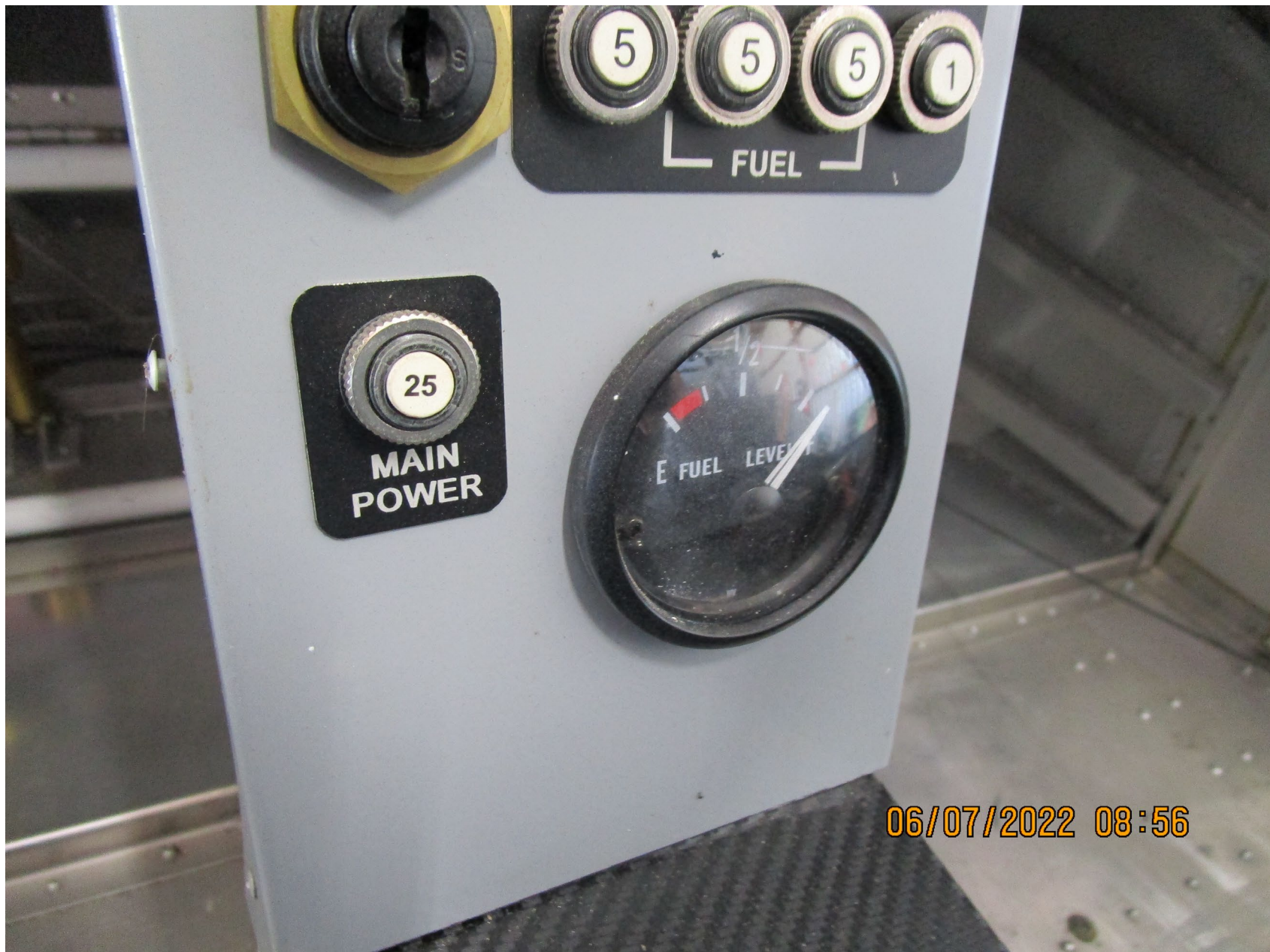
Photo 3 – Faulty fuel gauge (photograph provided by FAA)
