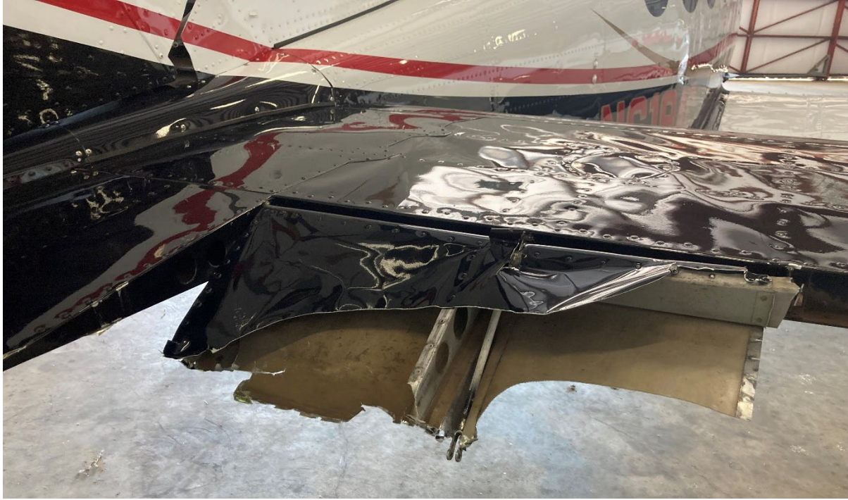
Figure 1. Right elevator partially separated.
