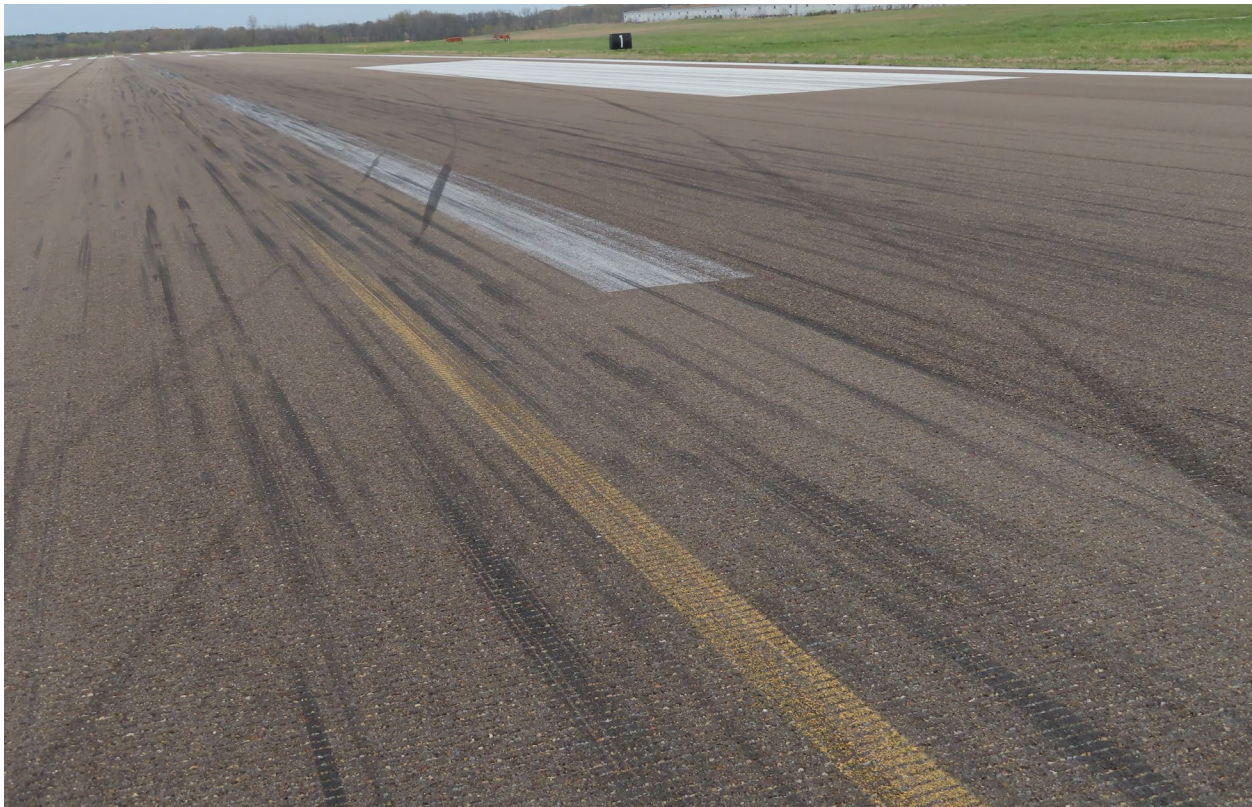
Figure 10. Rubber transfer marks on runway (viewed opposite direction of travel)
