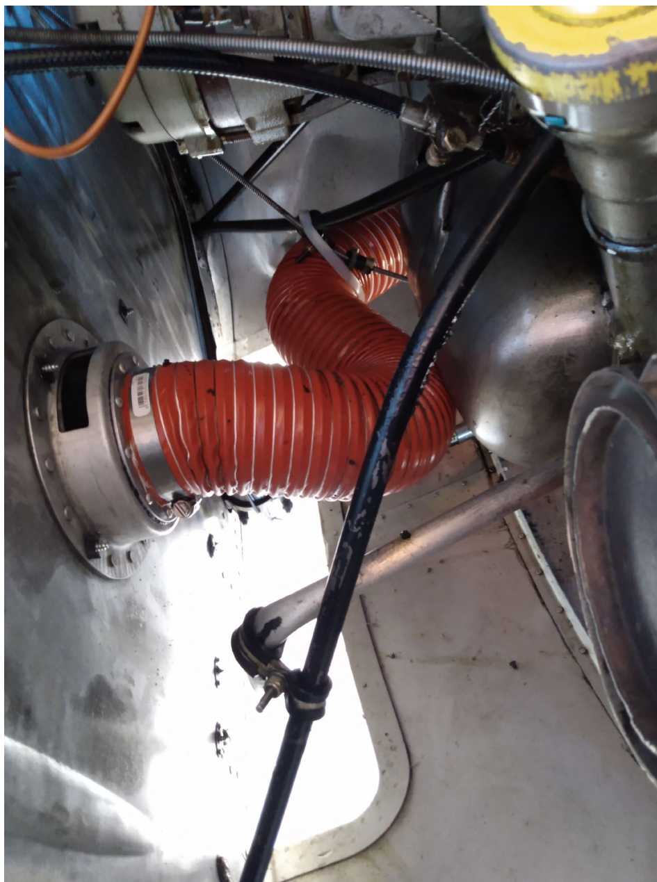
Photo 2 – View of bent engine mount tubes (Photo provided by FAA)
