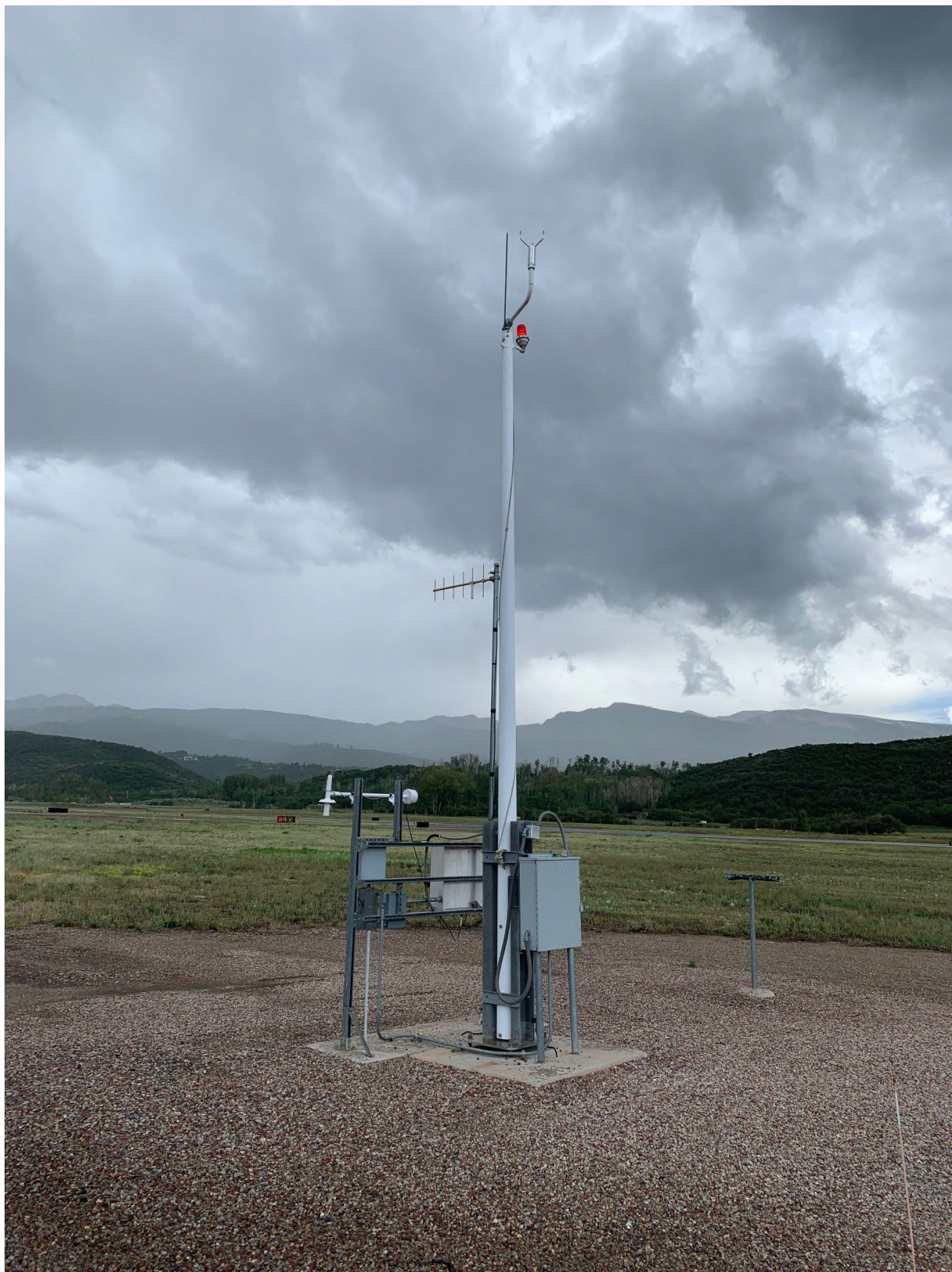
Figure 5. ASE SAWS equipment.
