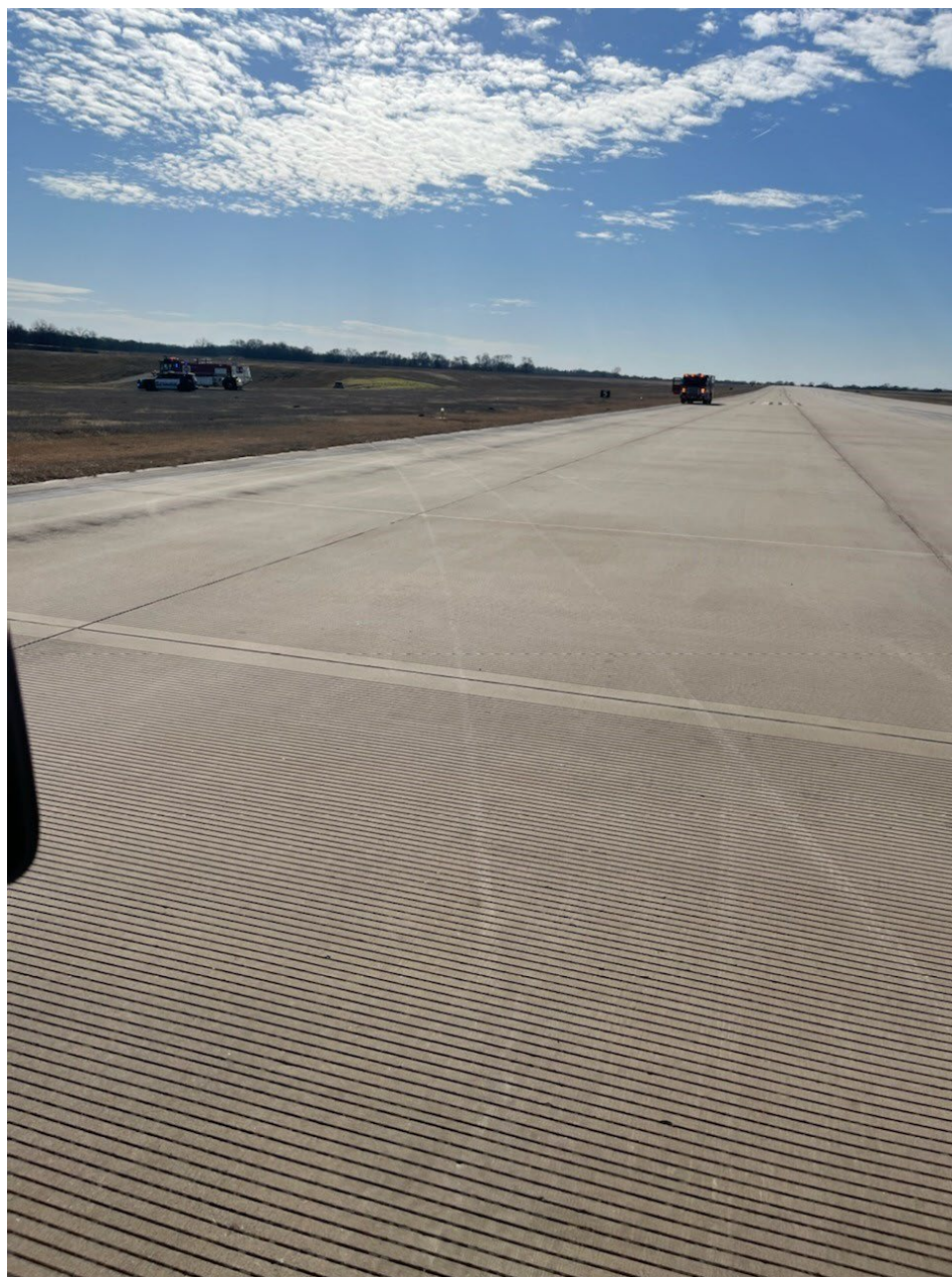
Photo 2 – Tire Marks Leading off Runway
