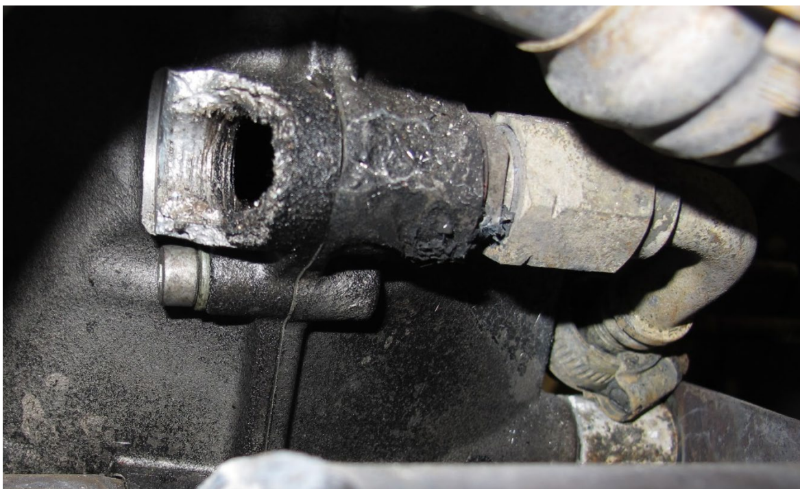
Figure 15. Closeup of frange connection on engine block.
