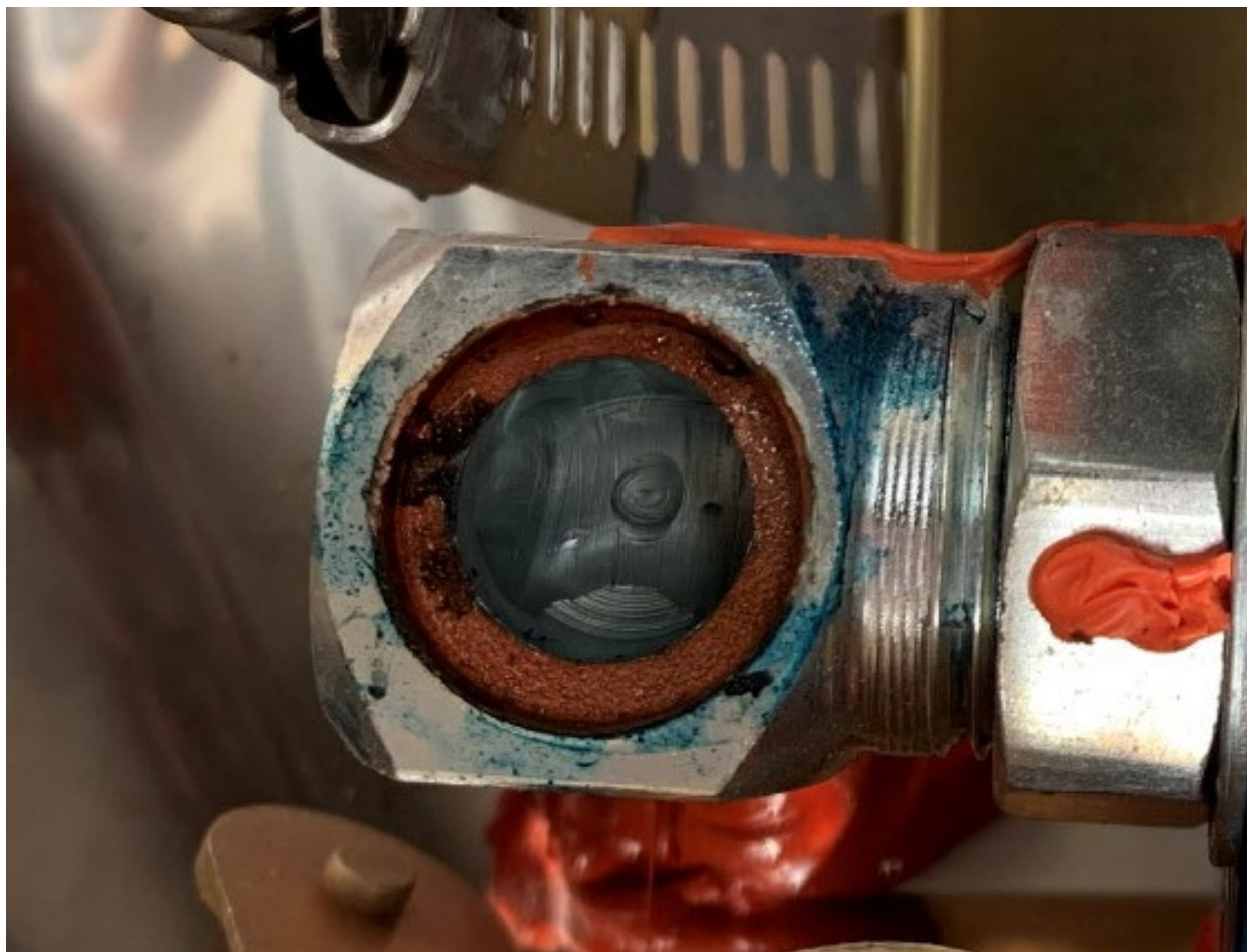
Figure 15. Excerpt of a photo taken during the wreckage exam showing the condition of the socket and surrounding surfaces at that time. Image courtesy of the investigator-in-charge.
