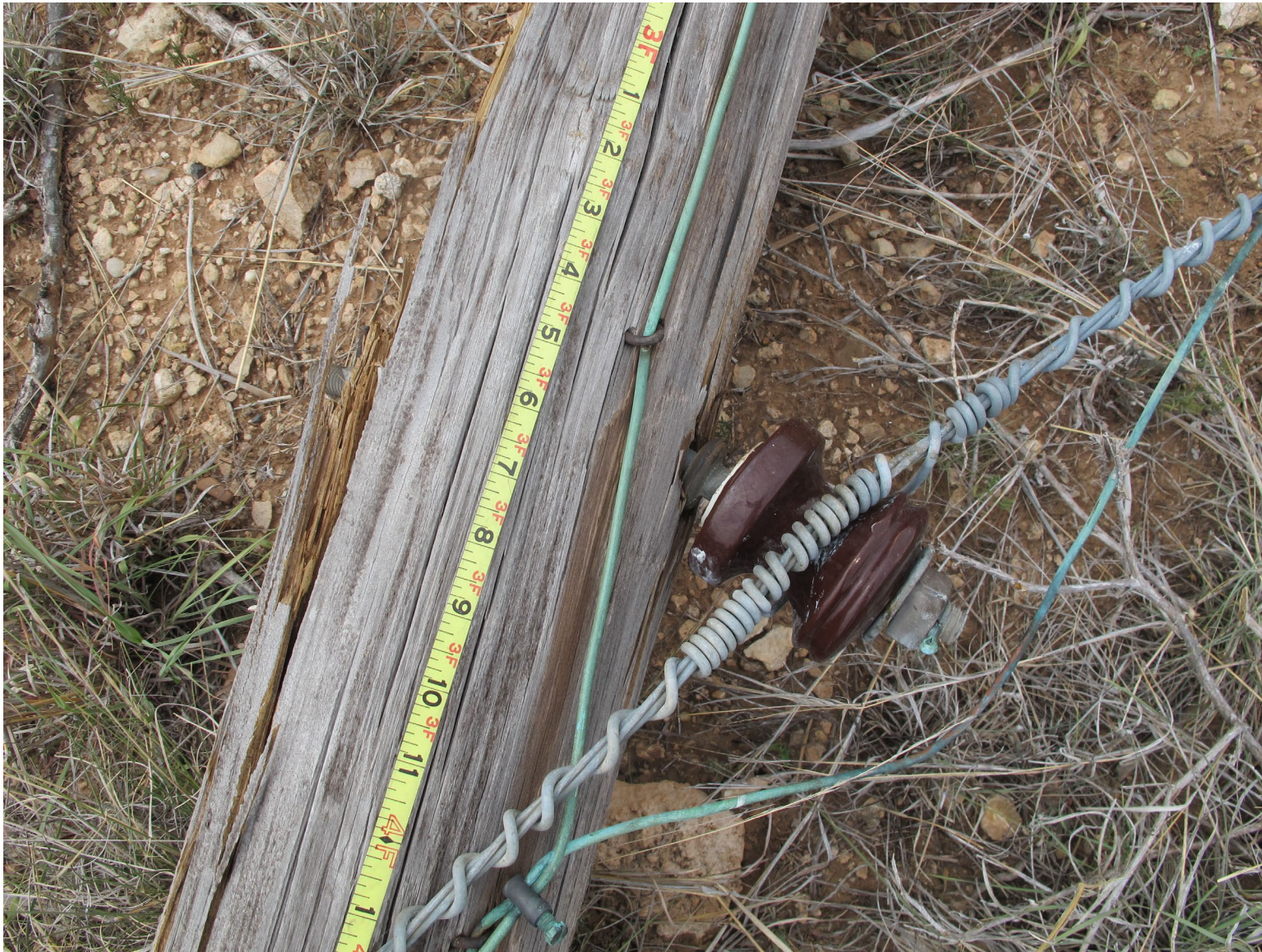
Photograph 8 - Closeup of Broken Pole and Wire (Courtesy of NTSB)
