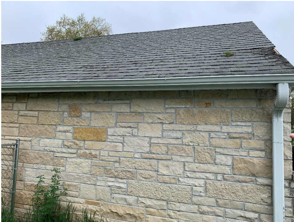
Figure 1: Damage to Garage Roof
