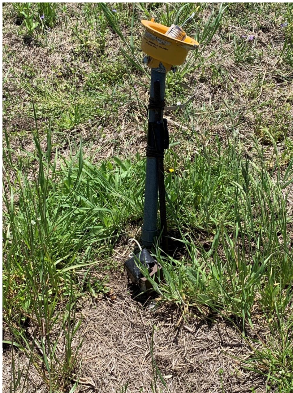
Photo 14 – Broken Runway Light
