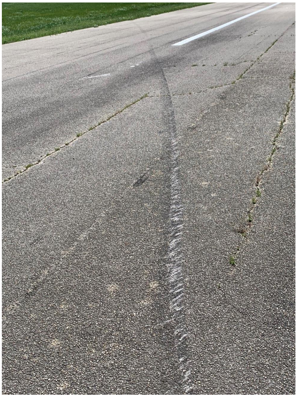
Photo 16 – Tire Marks in Detail
