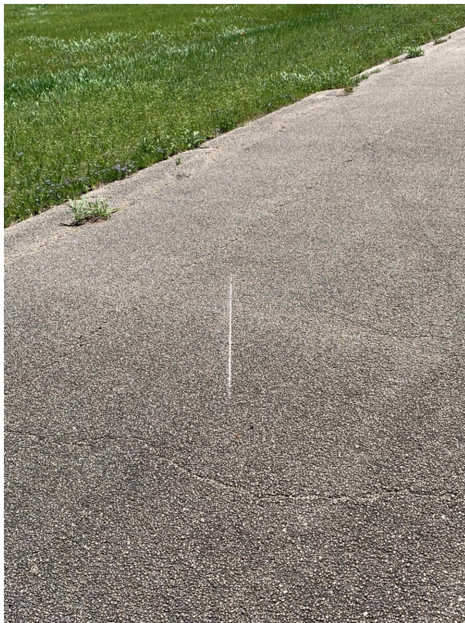
Photo 17 – Tail Tie-down Scrape in Runway
