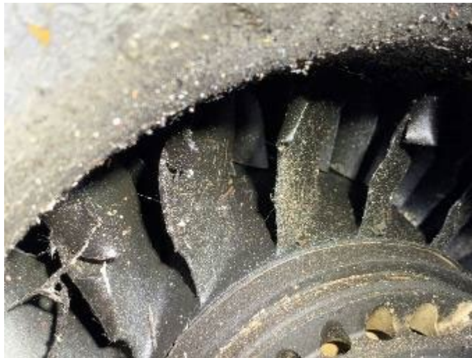
PHOTO 18: 1 ST STAGE COMPRESSOR DAMAGE
