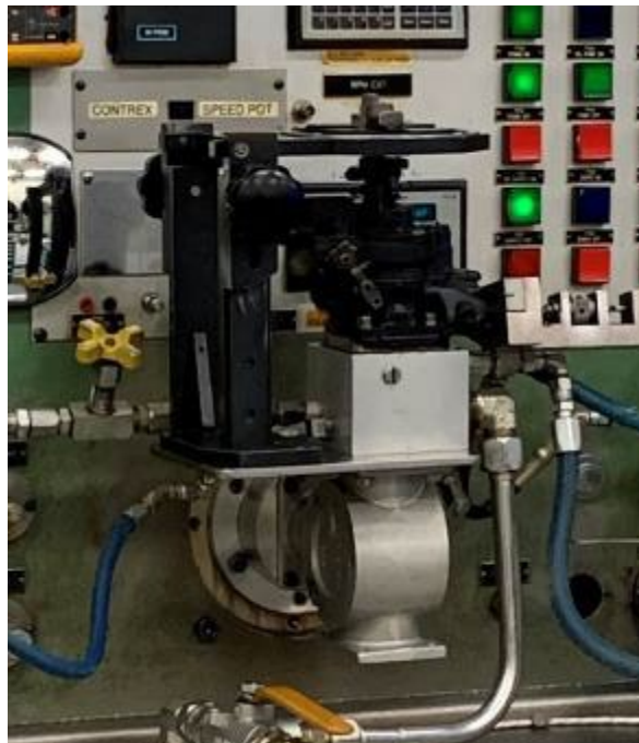
PHOTO 44: CSU ON THE WOODWARD TEST BENCH (COURTESY OF WOODWARD)
