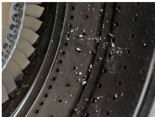
PHOTO 17: DEBRIS IN THE GAS PATH
