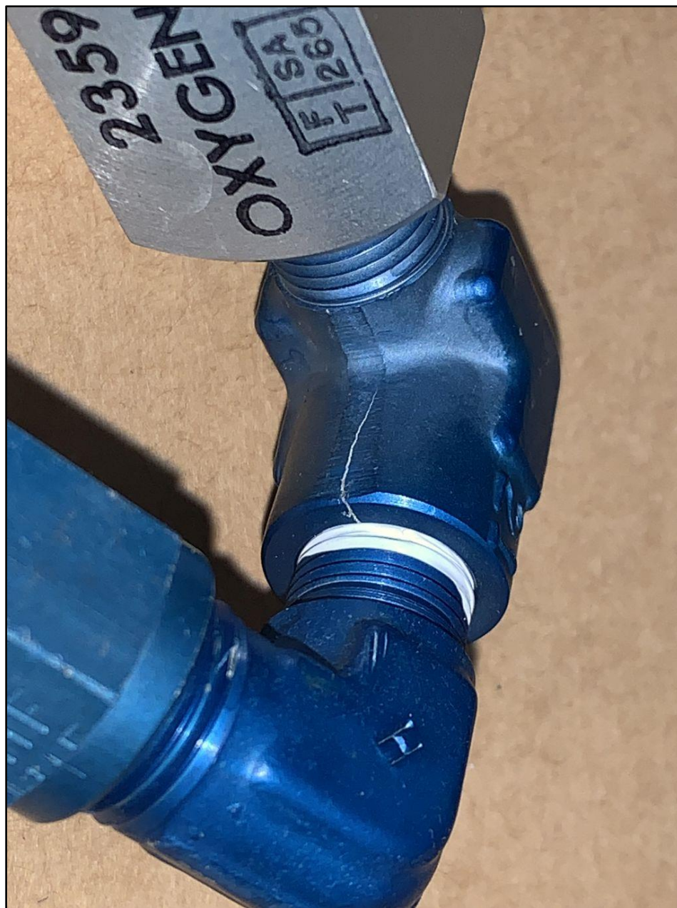
Photo 7 – Pilot-Side Oxygen Fitting
