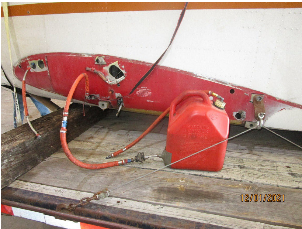
Figure 2: Fuel container – being plumbed into airplane's fuel system
