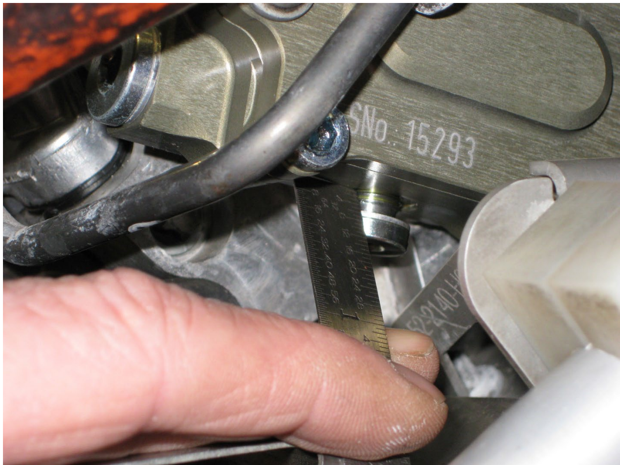
Right Engine Fuel Feed Pump prior to re-seating bolt.
