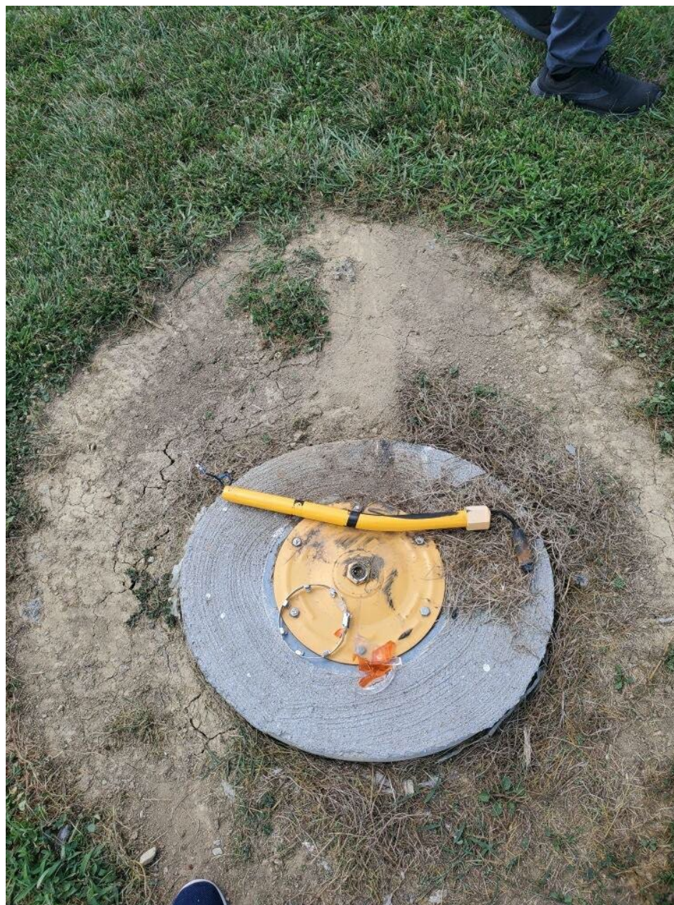
Photo 2 – Runway Light (FAA Photo)
