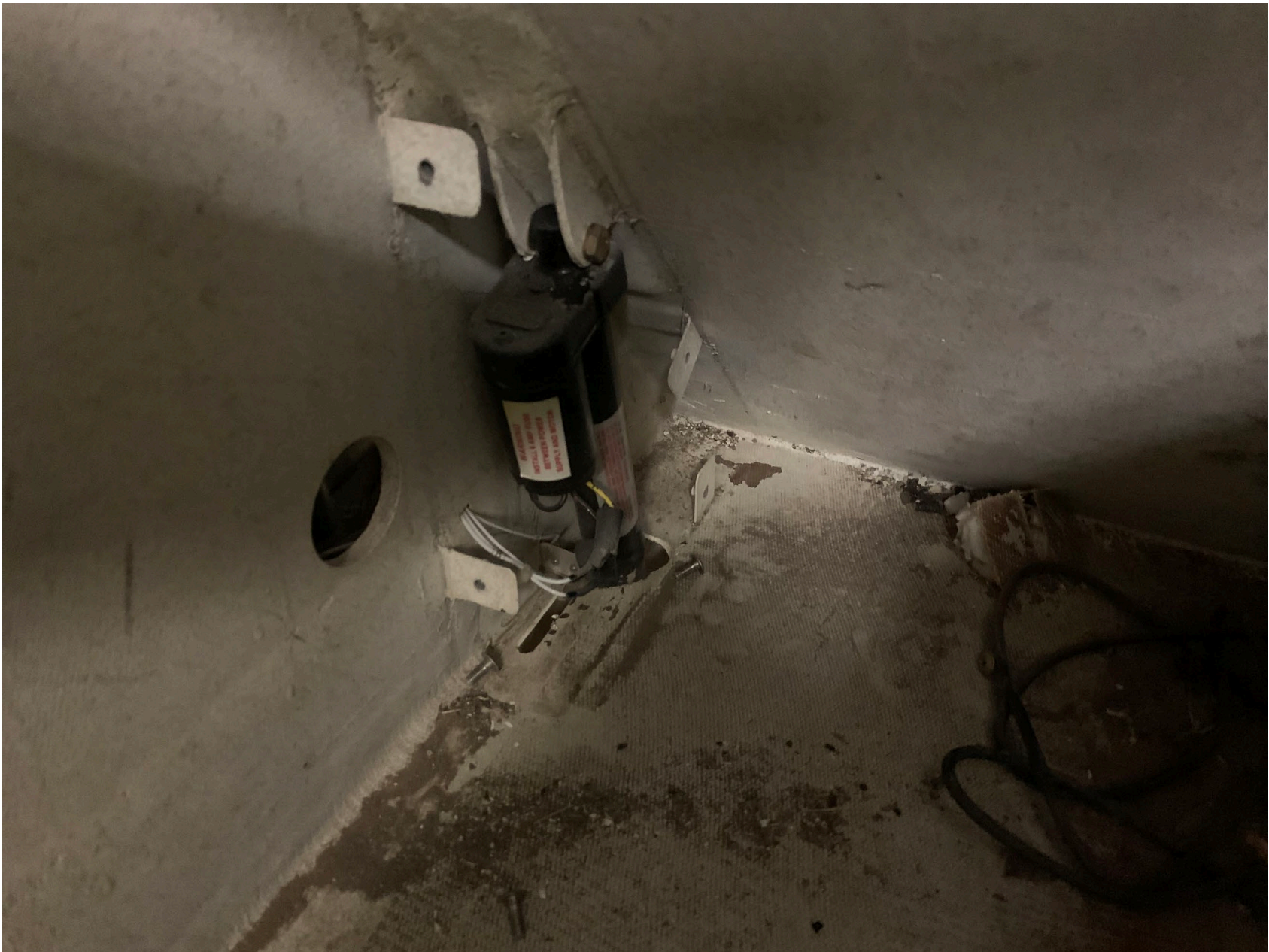
Photo 7 – View of the air brake actuator installed in the airframe.
