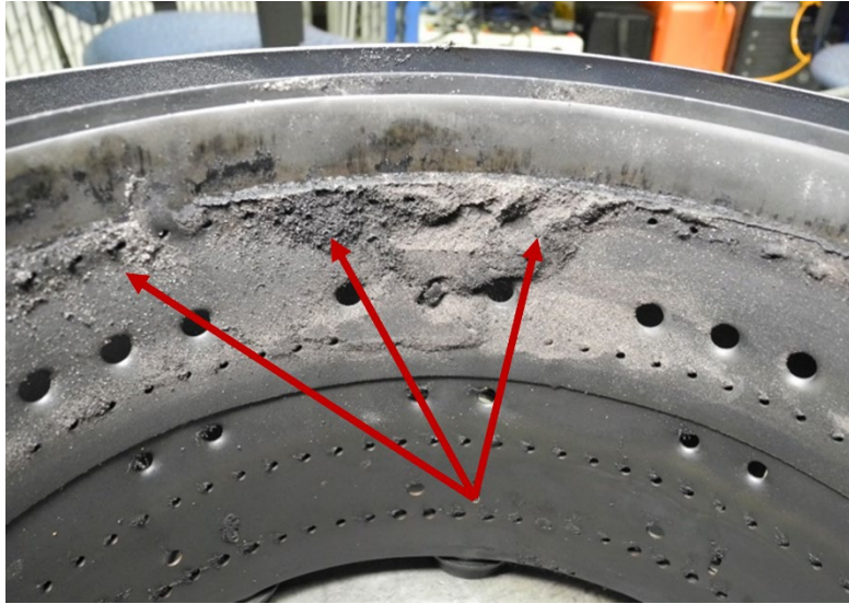
Photo 10: Burnt debris on the inner combustion liner.
