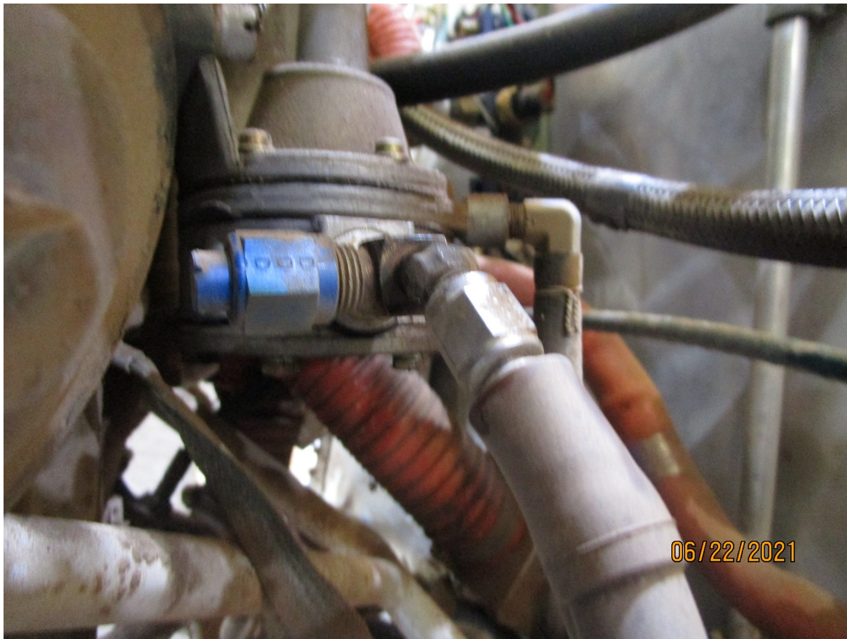
Photo 3 – Engine driven fuel pump
