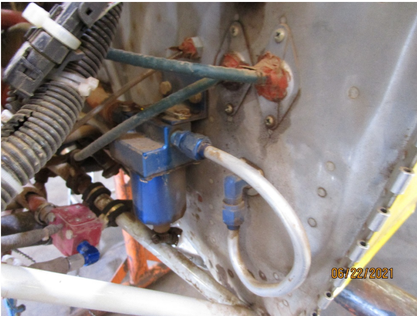
Fuel from tank thru gascolator, then to fuel pump
