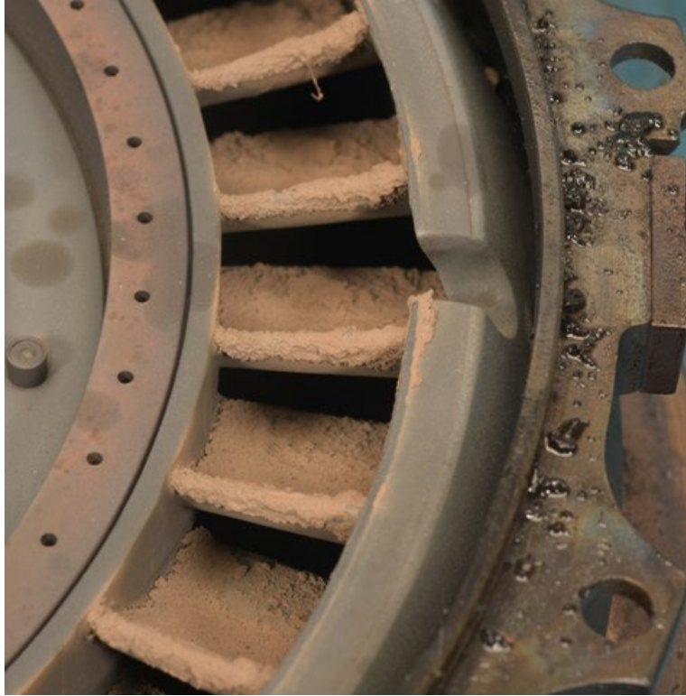
Photo 15- Earthen Debris on 1 st Stage Stator Vanes, Pressure Side/Leading Edge
