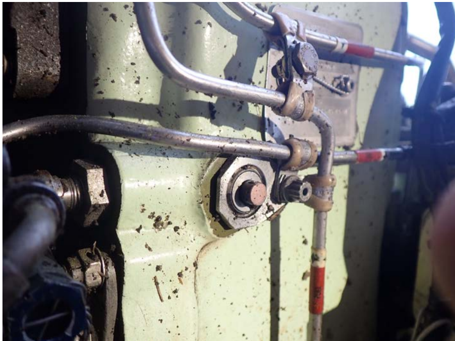
Figure 18. Engine S/N P-92143 Oil Filter Bypass Indicator
