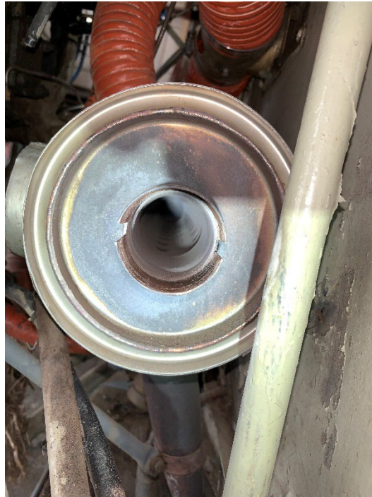
Photo 11: Internal View of Heat Exchanger
