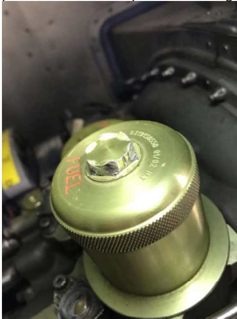
Fuel Filter Cap onsite
