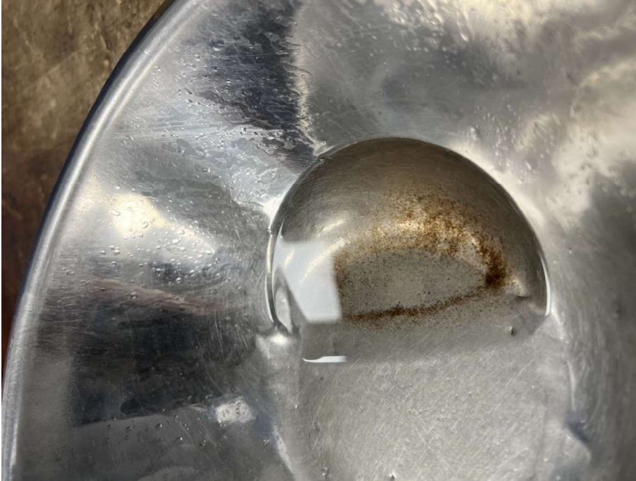
Contamination captured when FCU filter was removed
