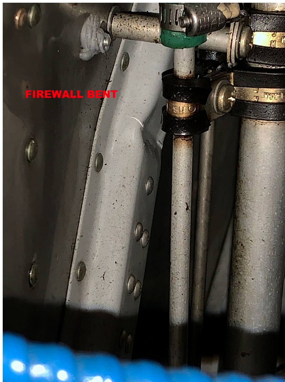
Photo 2 – Firewall Damage (FAA Photo)
