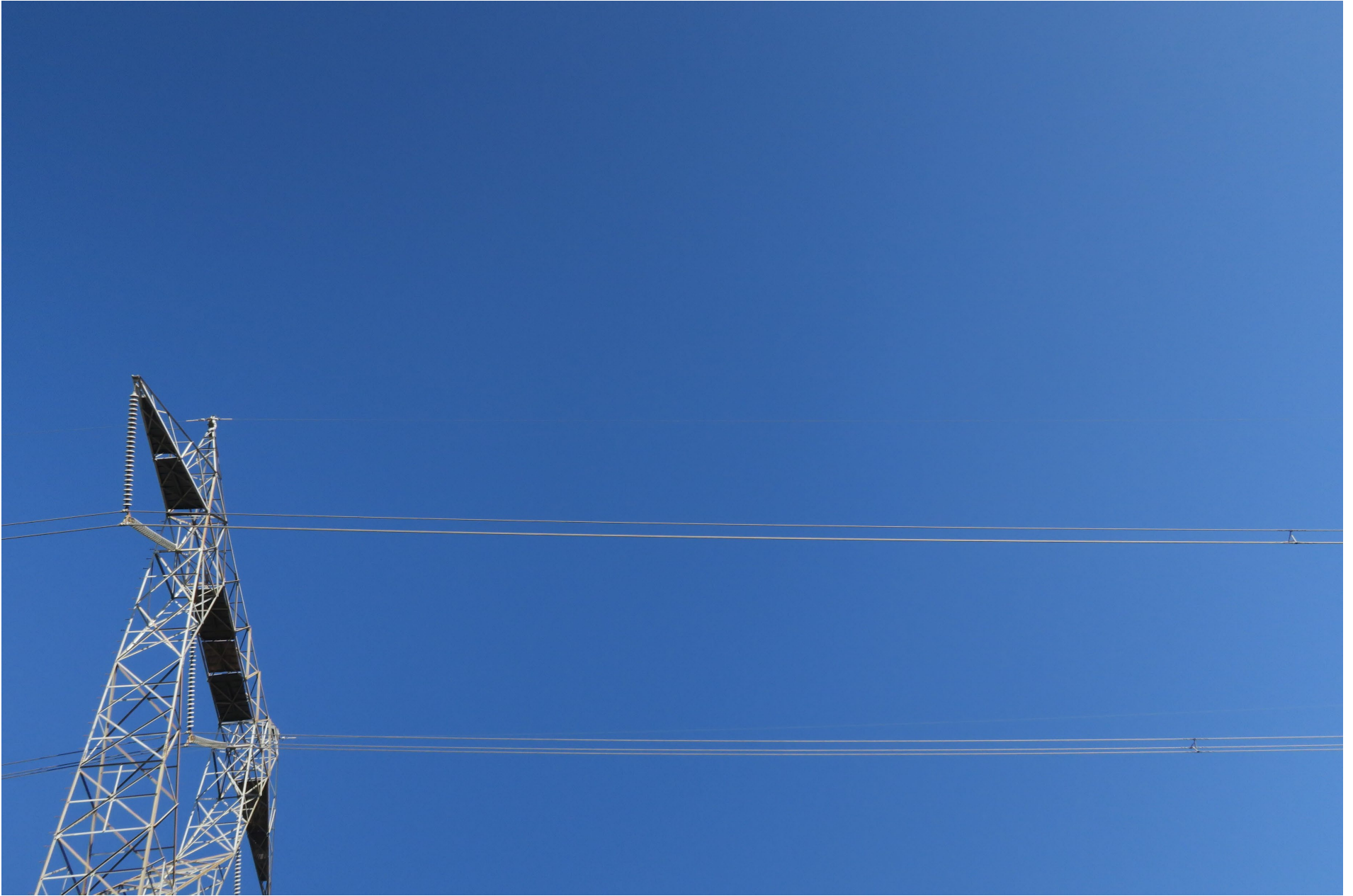
Photo 6 – View of the power lines at the accident site (courtesy of Textron Aviation).
