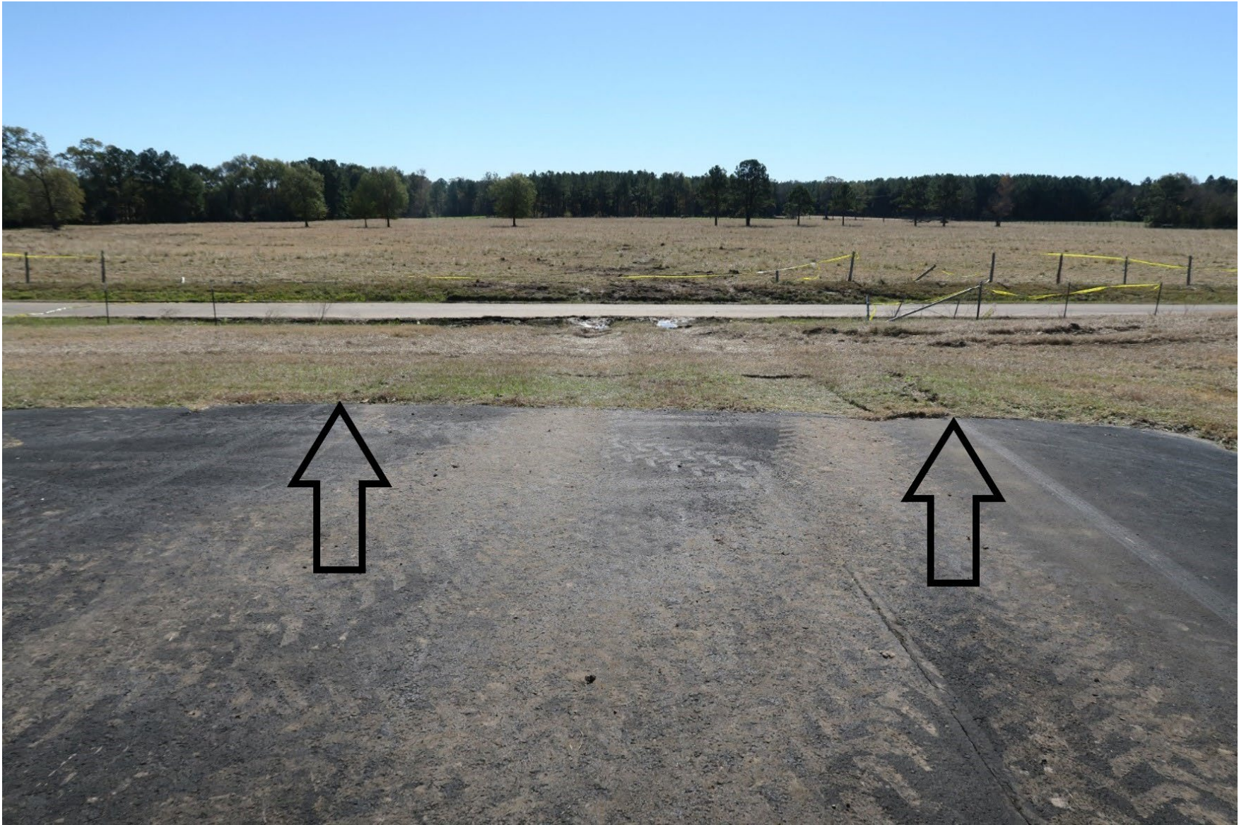
Photo 4 – Tires Marks at End of Runway 16 (Source: FAA)
