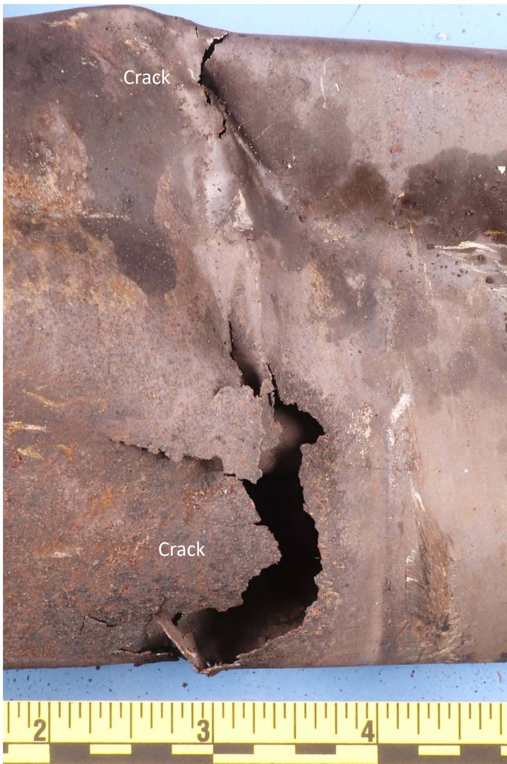
Figure 7 Cracks in muffler 2 in the main body of the outer shell.
