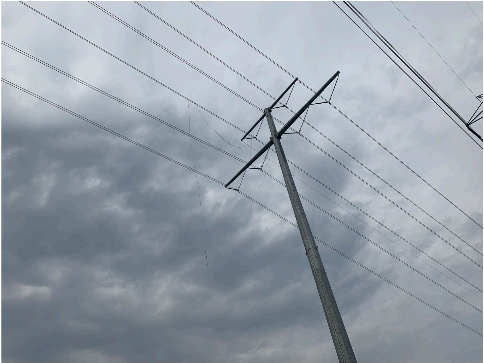
Photo 11 – View from underneath the transmission static lines, showing a transmission static line that was impacted by the airplane.
