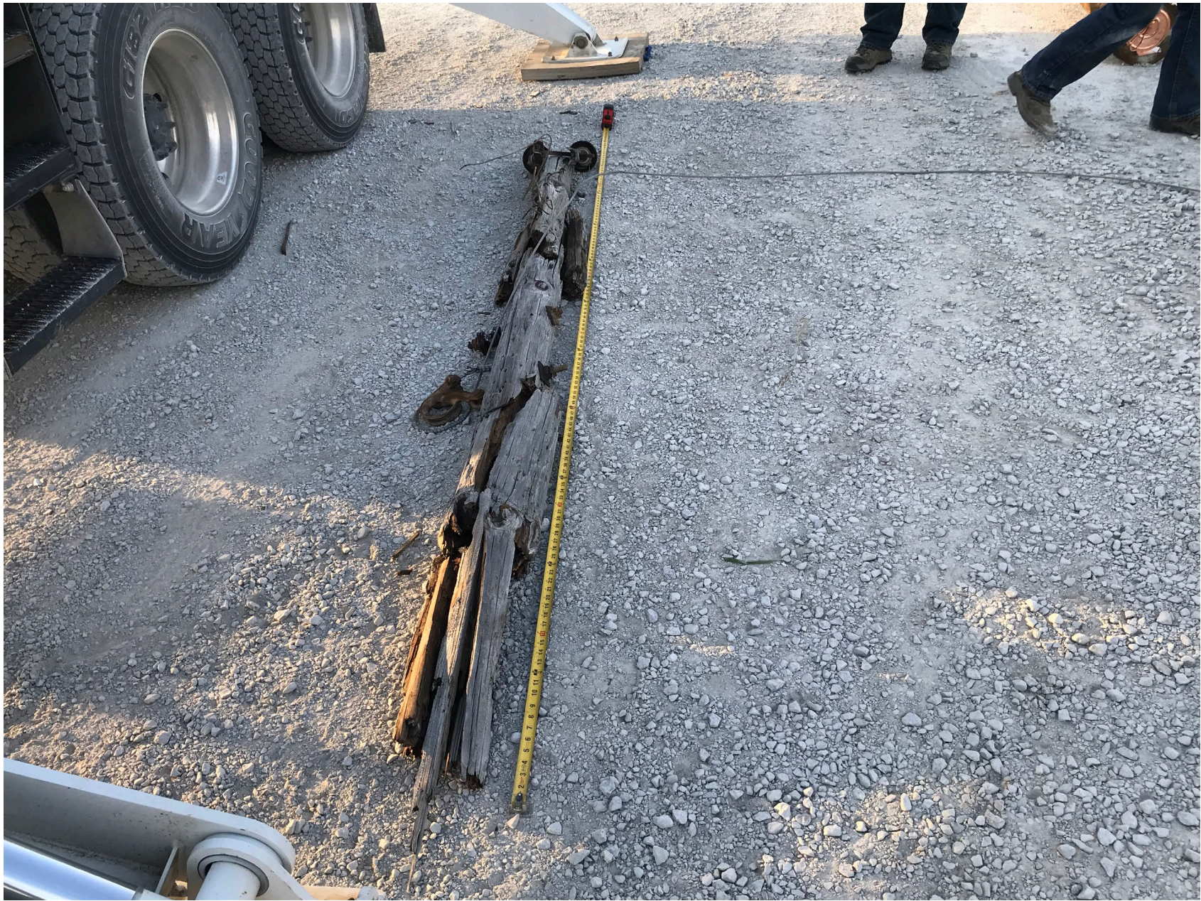
Photo 4 – Separated Power Pole (photograph provided by sheriff's office)
