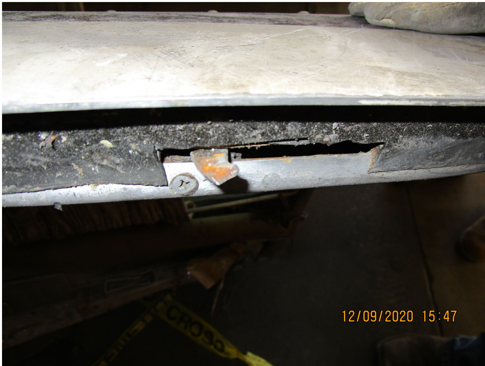
Photo 8 – Cabin door latch hook
