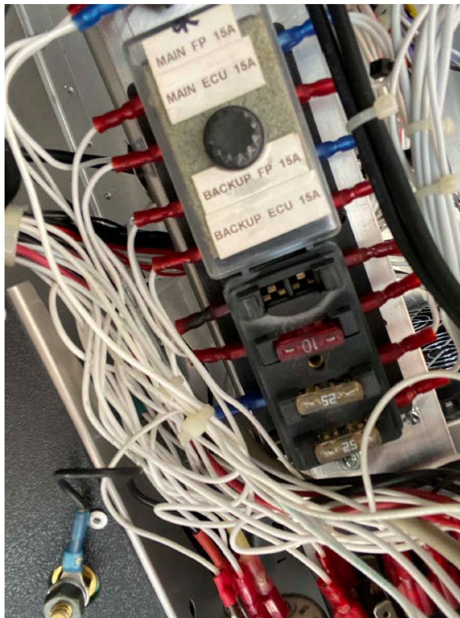
Photo 2 – Fuse Box (photo provided by Viking Aircraft Engines)
