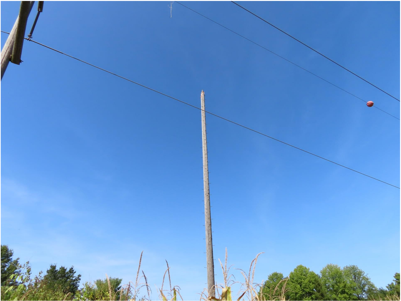
Photo 5 – Single Wood Pole Damage. Photo from Piper Aircraft
