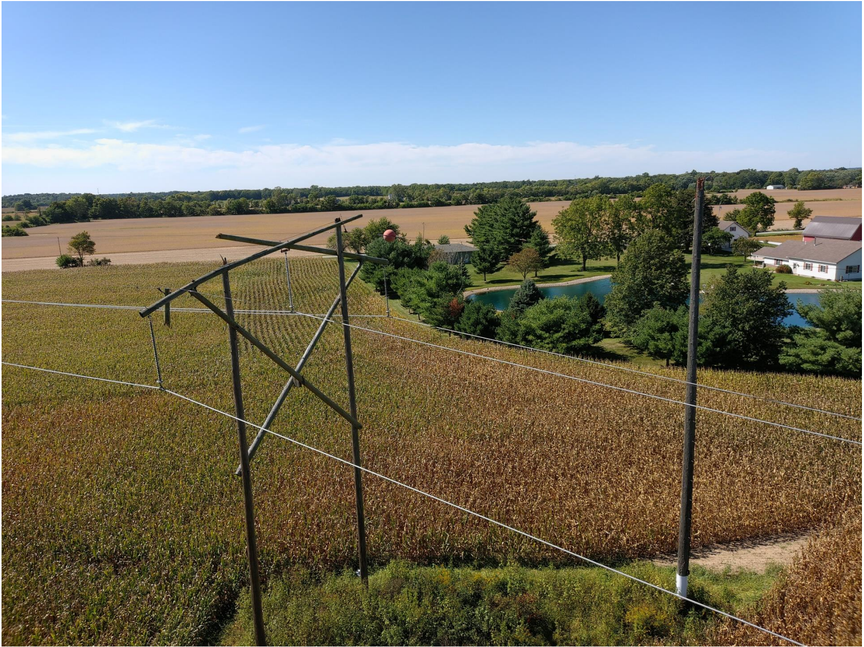
Photo 4 – Wood Pole and Dual Pole Utility Tower Damage, Photo from FAA
