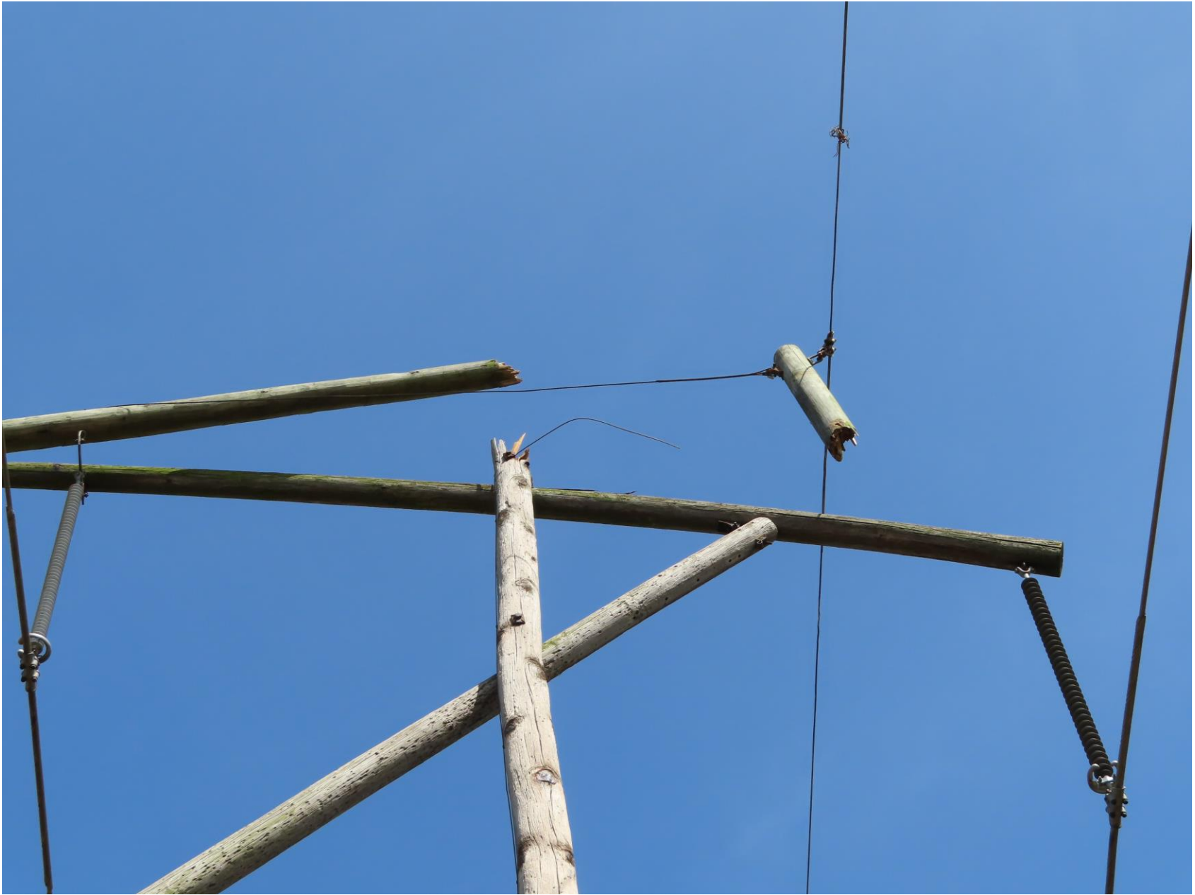
Photo 6 – Dual Pole Utility Tower Cross Pole Damage. Photo from Piper Aircraft.
